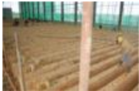
Interior of the coking oven: coking chambers
