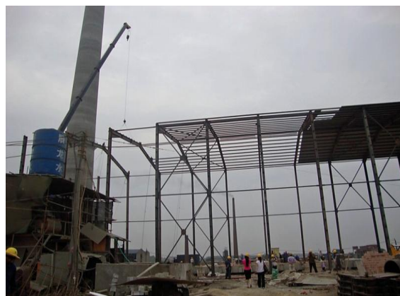
Main frame of the coking oven
